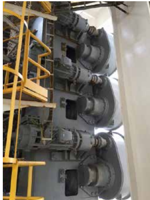
Jacking system units
